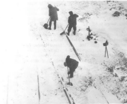
SHOVEL AND BROOM were used by these employees trying to release points of a switch so it could be thrown. Switch heaters could not melt snow as fast as it accumulated.
