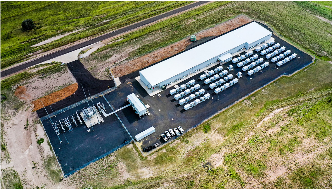
Example of Battery Energy Storage System Unit
