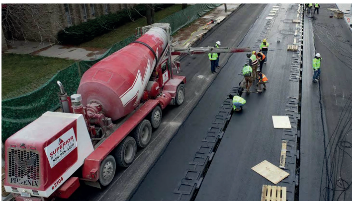
Workers filling trench and placing coils prior to paving on 14th Street
