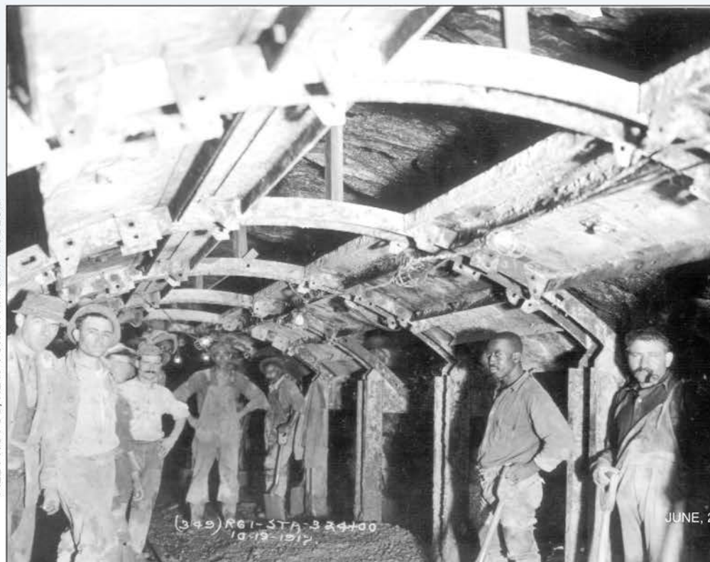
"Sand hogs" continue their work in the tunnel under Joralemon and Furman Streets. (60th Street Tunnel; 1919)
