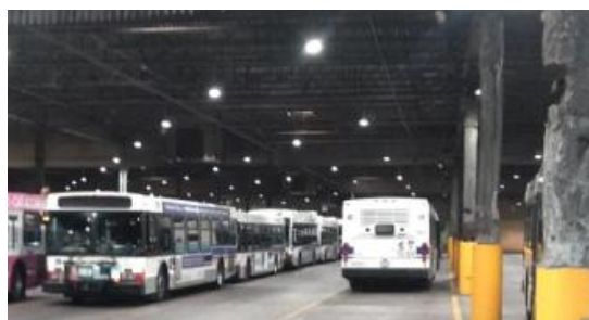
New LED lighting at CTA's Chicago Bus Garage
